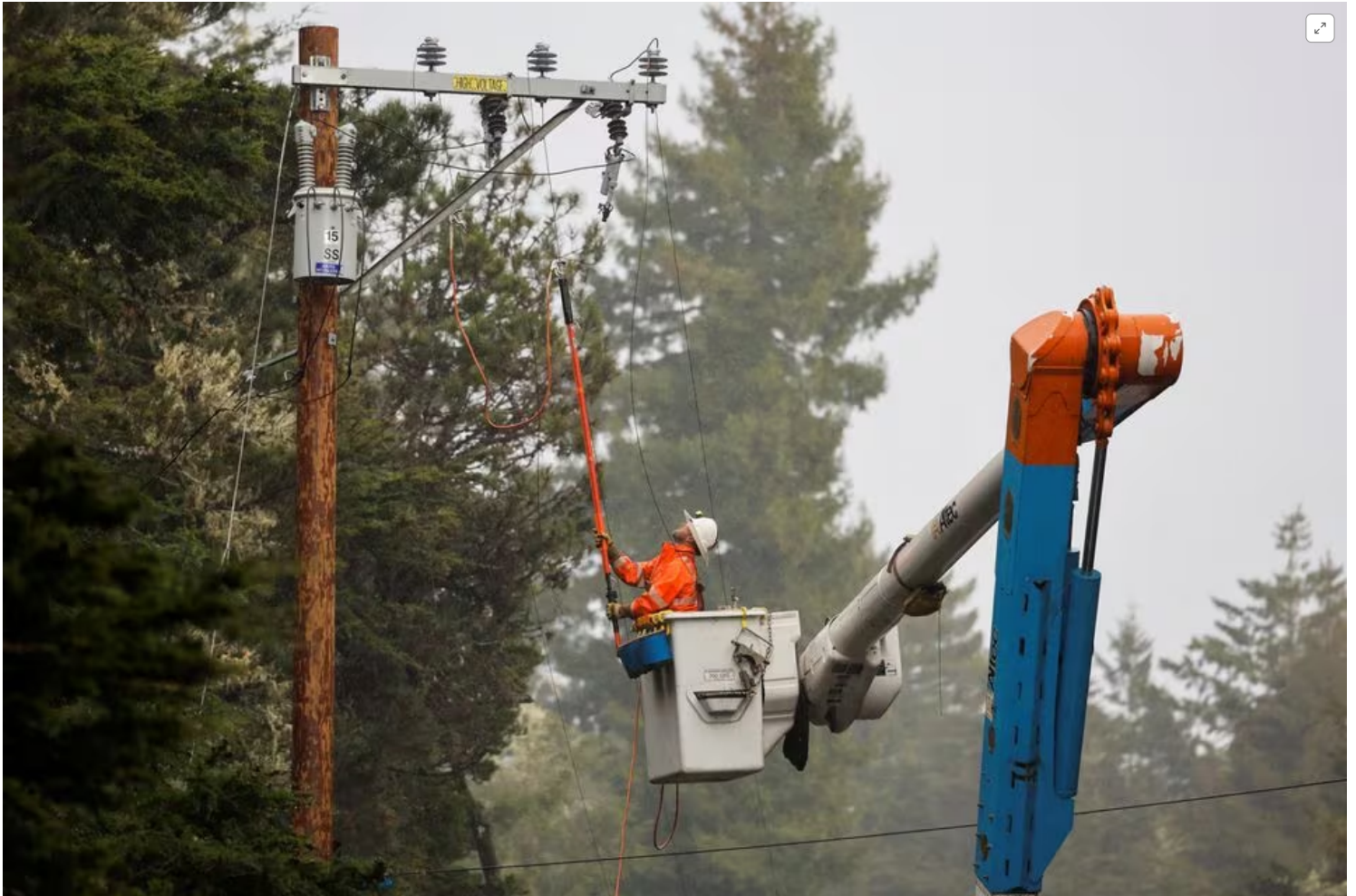
[1/6] A member of a Pacific Gas & Electric crew works to repair a power line, following storms in Mendocino, California, U.S. January 5, 2023. REUTERS/Fred Greaves Acquire Licensing Rights
