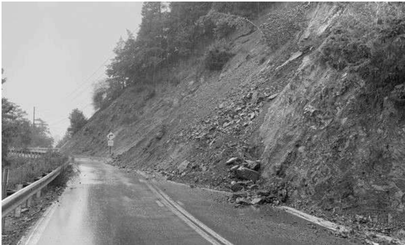
An active slide blocking Route 271 near Big Bend Lodge Road [PM 2.68] in Mendocino County, Calif., on Feb. 4, 2025. (Courtesy: Caltrans)
